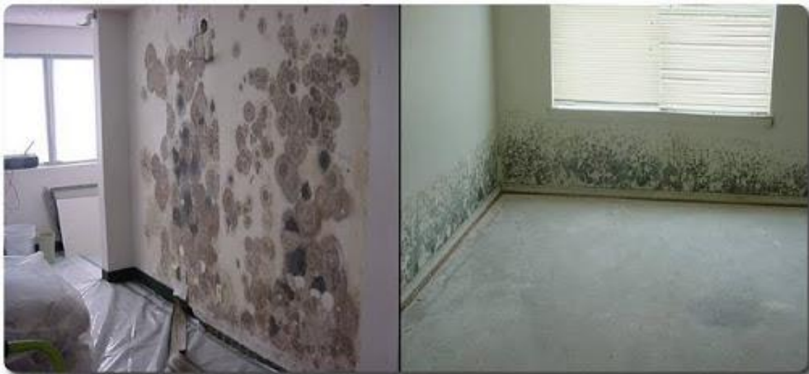
Mold on interior walls. On left, mold formed behind wallpaper. On right, mold from water intrusion after flood/floor moisture.
